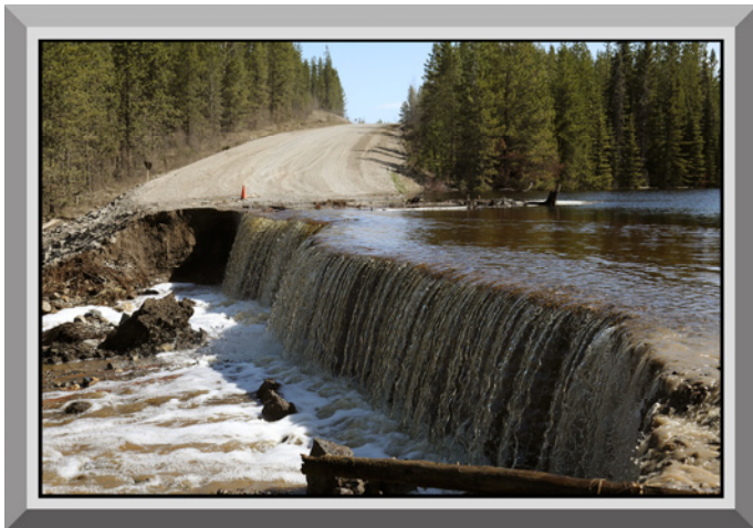
Figure 4.20 Be Wary of Road Washouts.
