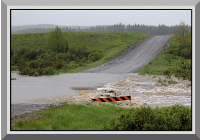
Figure 4.19 Unsafe Water Crossing.
